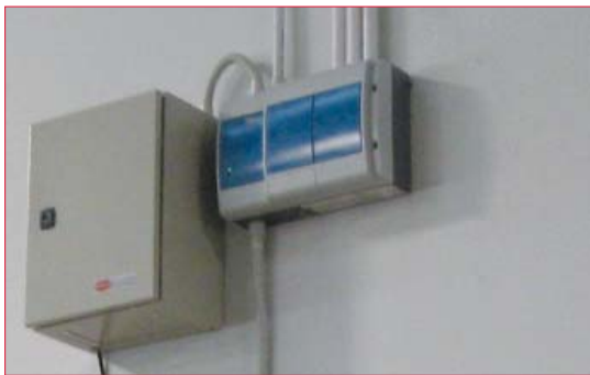
Direct connection from the Xtralis VESDA detector to the existing security panel met the insurer's requirements.
